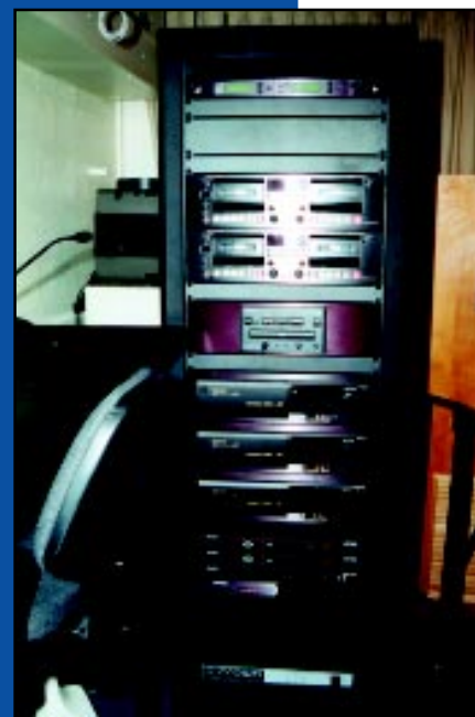
The Middle Atlantic rack is positioned so the operator has easy access to the AV controls as needed during presentations.
